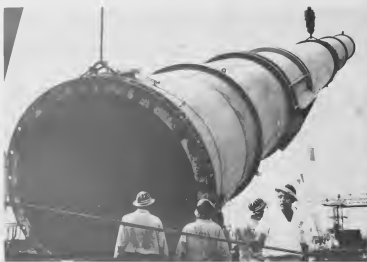
AS RIGGER Foreman L. F. Moritz, foreground, calls out orders, the guyed derrick pulls the 180-foot stack off the ground. The cable around the boom keeps the thirteen-cable block, and load, directly under the derrick's boom.
